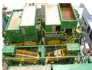
1800m 3 /hr Slurry Treatment Plant, Singapore
