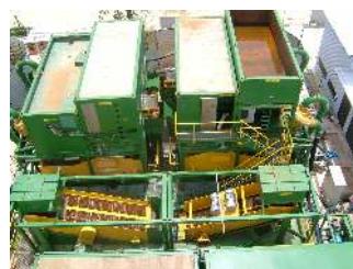
1800m 3 /hr Slurry Treatment Plant, Singapore
