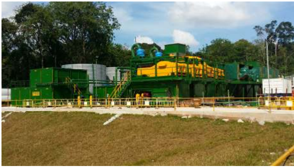
2x1400m 3 /hr Slurry Treatment Plants, Singapore
