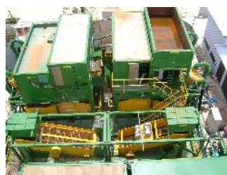
1800m 3 /hr Slurry Treatment Plant, Singapore
