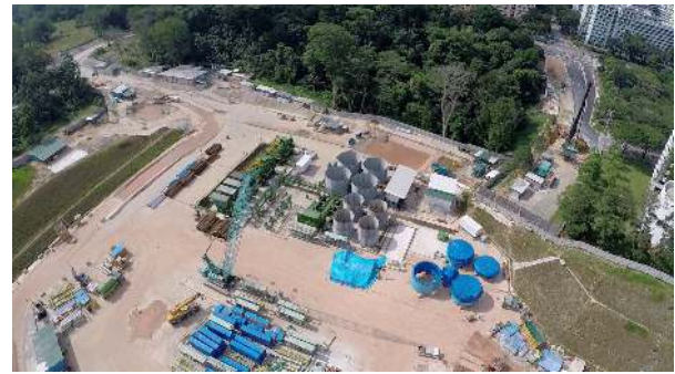
2x1000m 3 /hr Slurry Treatment Plants, Singapore
