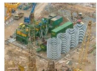
1350m 3 /hr Slurry Treatment Plant, Kowloon, Hong Kong
