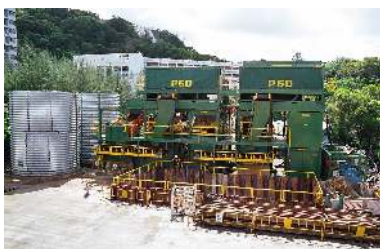
800m 3 /hr Slurry Treatment Plant, Kai Tak, Hong Kong
