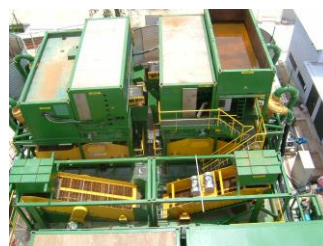
1800m 3 /hr Slurry Treatment Plant, Singapore
