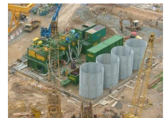
1350m 3 /hr Slurry Treatment Plant, Kowloon, Hong Kong
