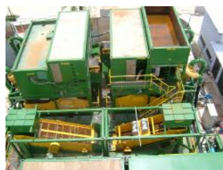
1800m 3 /hr Slurry Treatment Plant, Singapore
