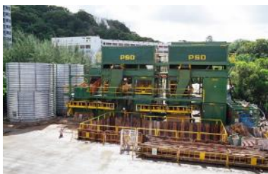
800m 3 /hr Slurry Treatment Plant, Kai Tak, Hong Kong
