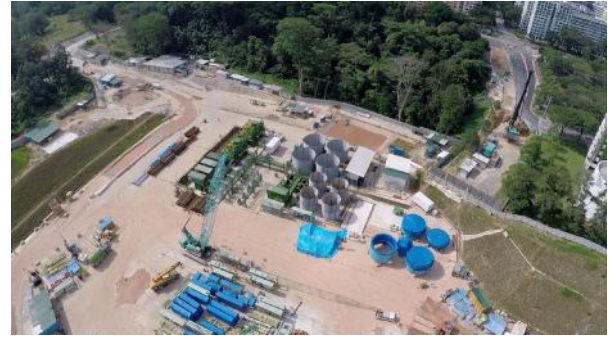
2x1000m 3 /hr Slurry Treatment Plants, Singapore
