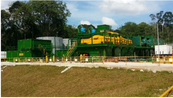
2x1400m 3 /hr Slurry Treatment Plants, Singapore
