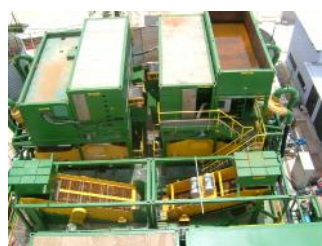
1800m 3 /hr Slurry Treatment Plant, Singapore
